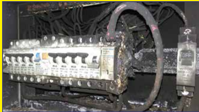
Make sure you get your switchboard and electrical equipment checked for safety before it's too late.
